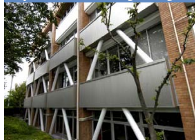
Earthquake resistant strengthening brace
